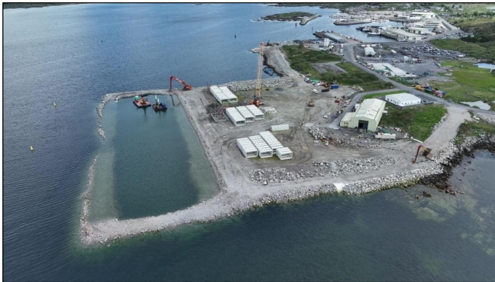
Figure 2-11: Site Status on 14 May 2024 when the presumed lawful works ceased.
