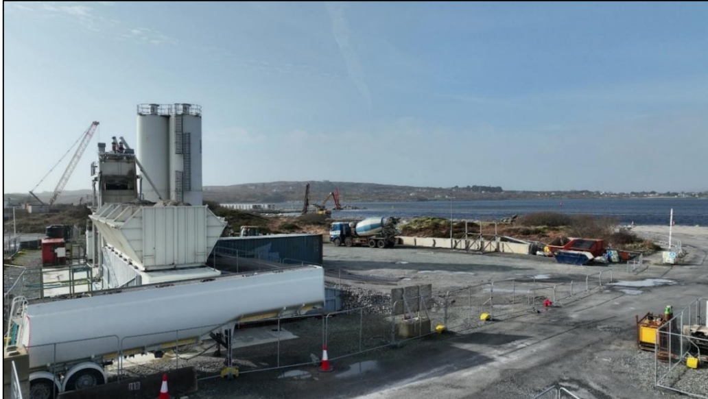
Figure 2-27: Photograph of the mobile Concrete Batching Plant and water storage tank.
